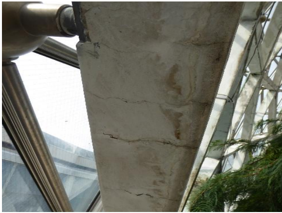
Figure 18. Transverse cracks on precast member
